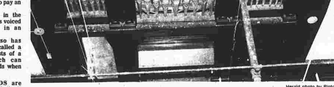
These pipes are what remains of the organ that used to be in Cheney Hall. The organ, in a state of disrepair, couldn't be restored, theater organ society representatives say.
